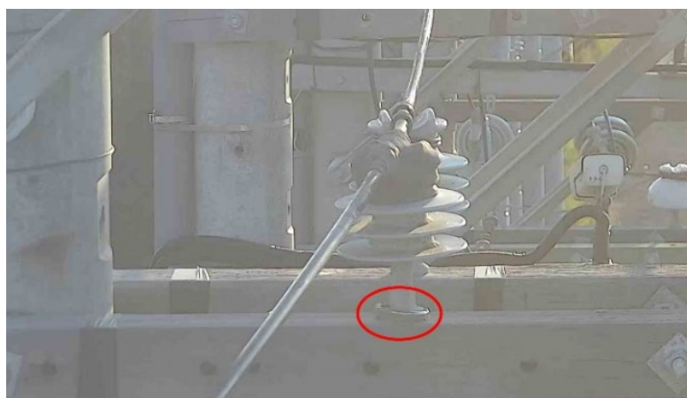
Figure 2. Collecting the leakage current surges of 15 kV HDPE insulator in the natural environment.
