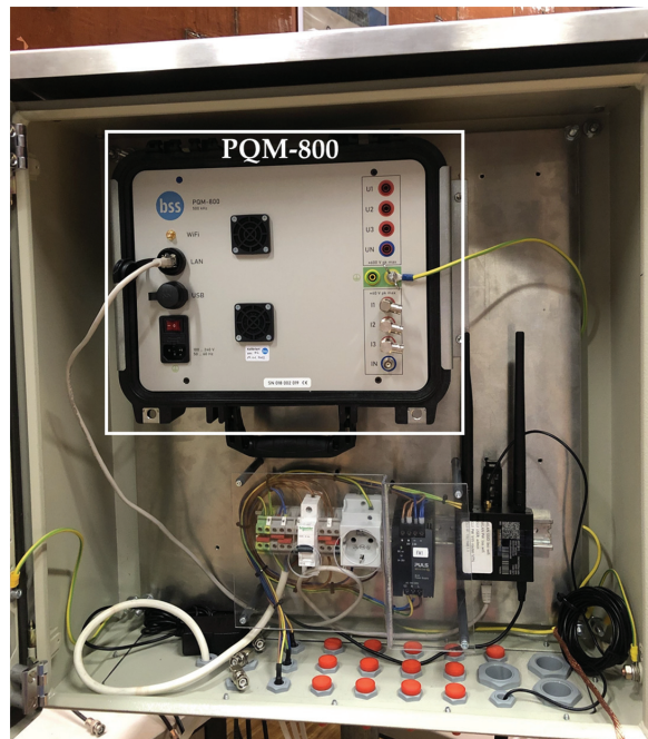
Figure 5. The control cabinet with the power quality monitor.
