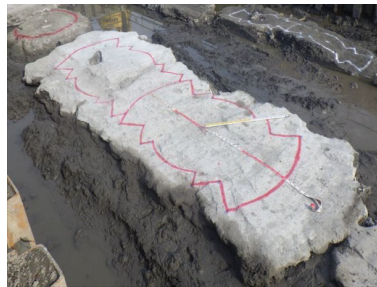
Figure 10. Rectangular-shaped stabilized soil column constructed via jet grouting method (courtesy of the Chemical Grouting Co., Ltd.).
