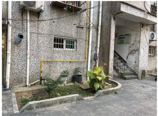
Stormwater planter in Yanyu Residence, Jiaying
