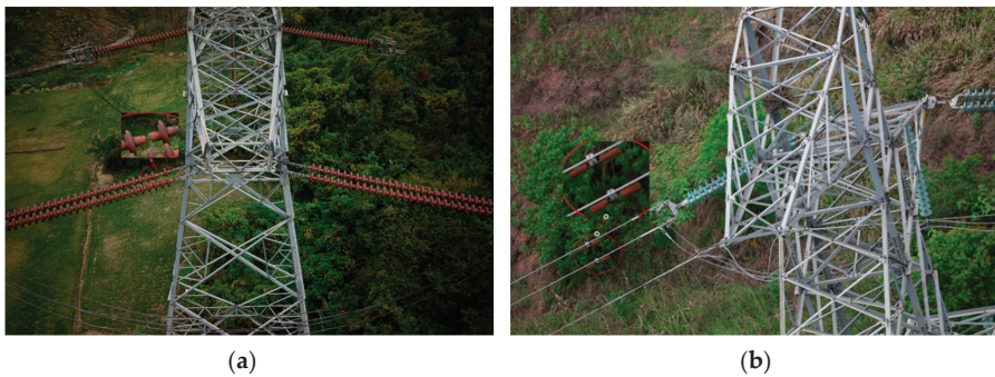
Figure 10. (a) Example of a broken insulator in a small target; (b) example of vibration hammer rust in small targets.
