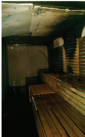
Figure 12. Bench and plywood boards at the ceiling and against the walls at the end of Test no. 7.
