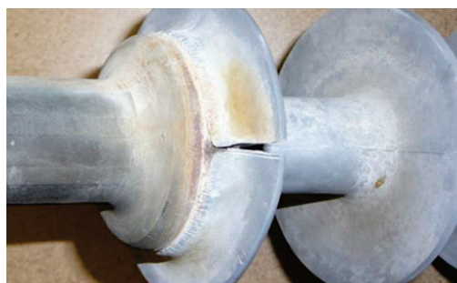
Figure 2. Deteriorated insulators that can be found by visual inspection [11].
