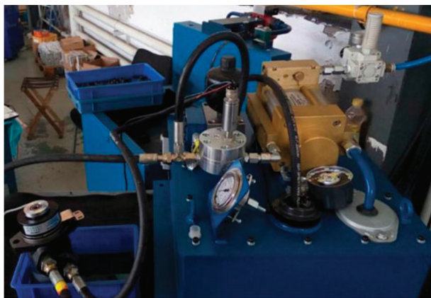
Figure 4. Dedicated test bench for the HP transformer.
