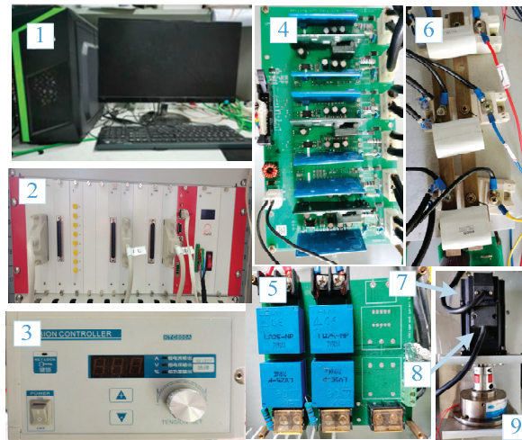
1-Computer 2-Controller 3-Tension controller 4-Driving circuit board 5-Current measurement circuits 6-Inverter 7-PMSM 8-Position sensor 9-Magnetic particle brake
