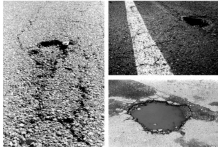
Figure 2. Moisture-induced pavement distresses.
