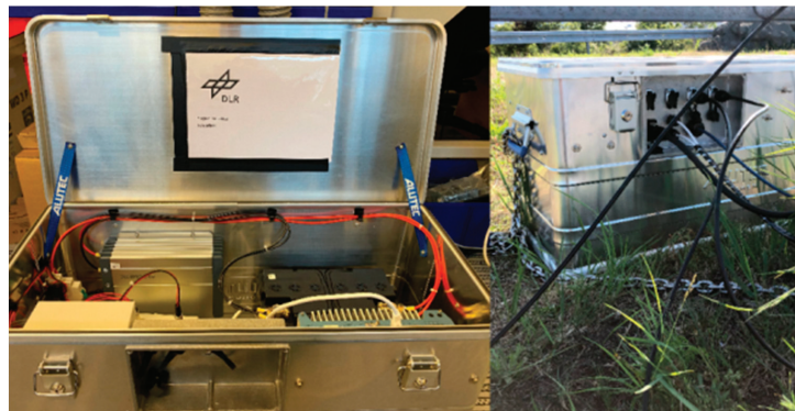
Figure 6. Sensor processing unit with battery backup that records the data from the LiDAR sensors together with various other sensors, such as AIS, camera, and weather-related information, and also communicates processed information via the mobile network.
