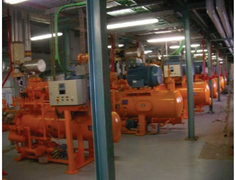
Figure 5. View of industrial refrigeration compressor room under study.
