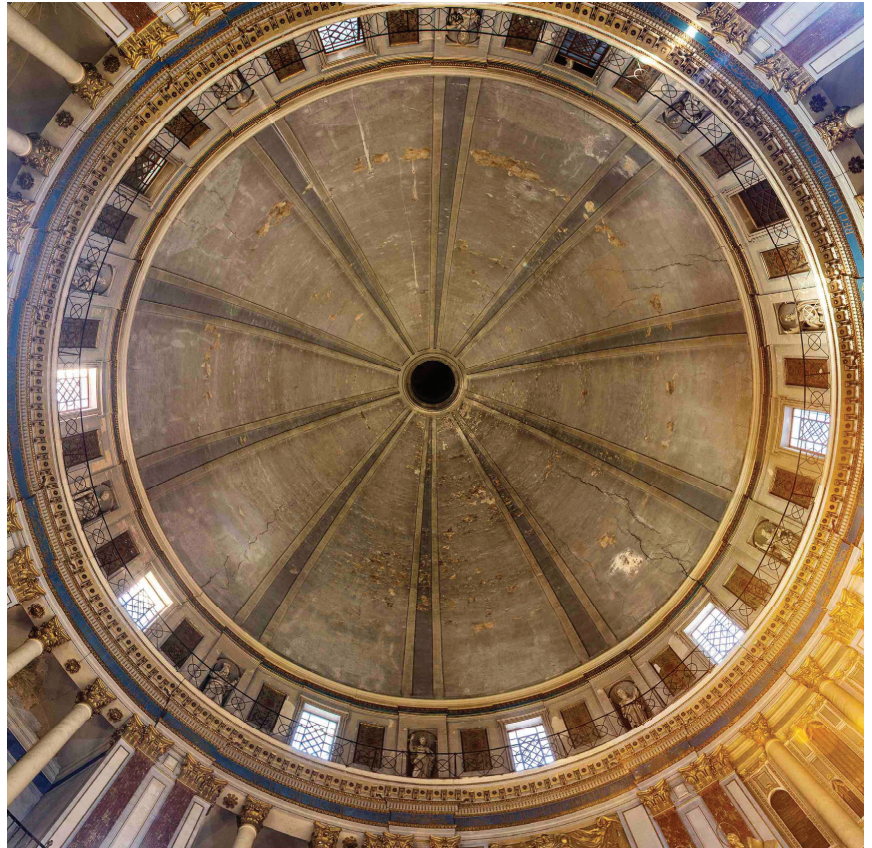
Figure 3. View of the dome and the cracks in four different sectors.
