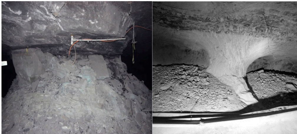
Figure 5. Views of damaged mine workings with inclined sidewall surfaces: (left) —long pillar at an intersection in Rudna mine, (right) —sidewall of a rectangular gallery with inclusion of competent rocks—Polkowice-Sieroszowice mine after blasting works in the close neighborhood, February 2016.
