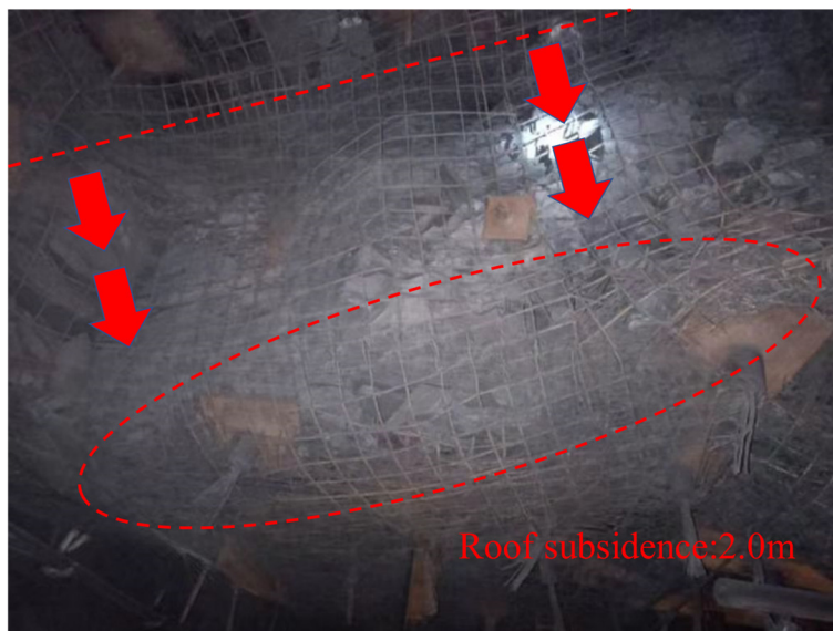
Figure 4. Subsidence of Roadway Roof.
