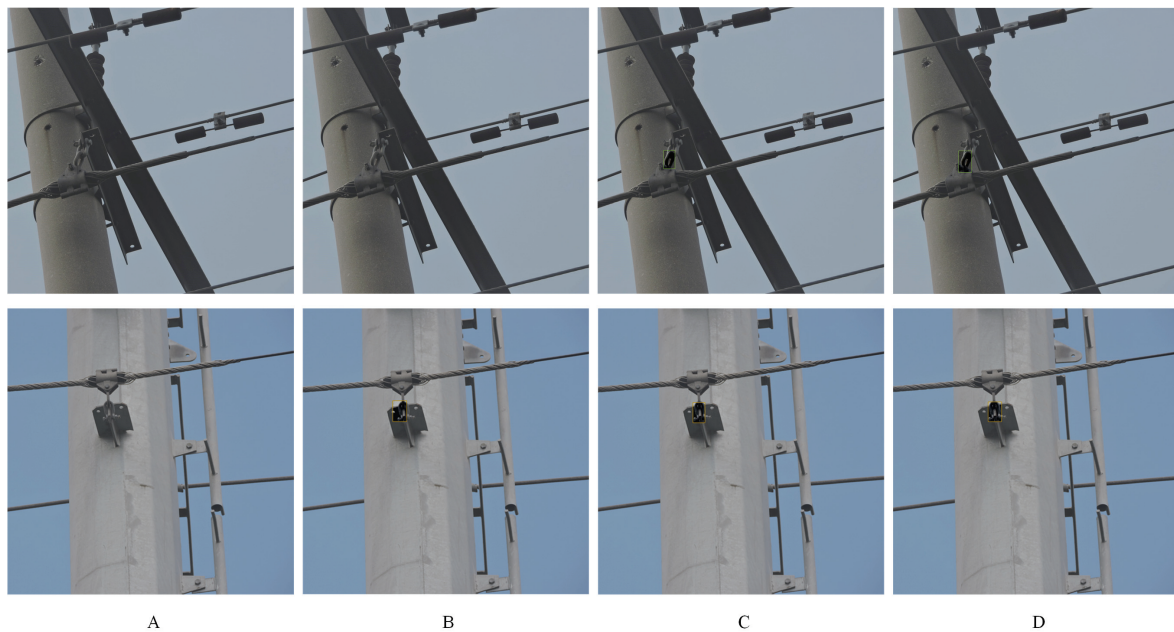
Figure 8. Visual detection results of small target fittings under various methods. The first and second rows depict the visual inspection results of a ball eye and a shackle, respectively. A is the U-Net, B is the U-Net combined with the DGCNN, C is the BRA-UNet, and D is the UD-Net.
