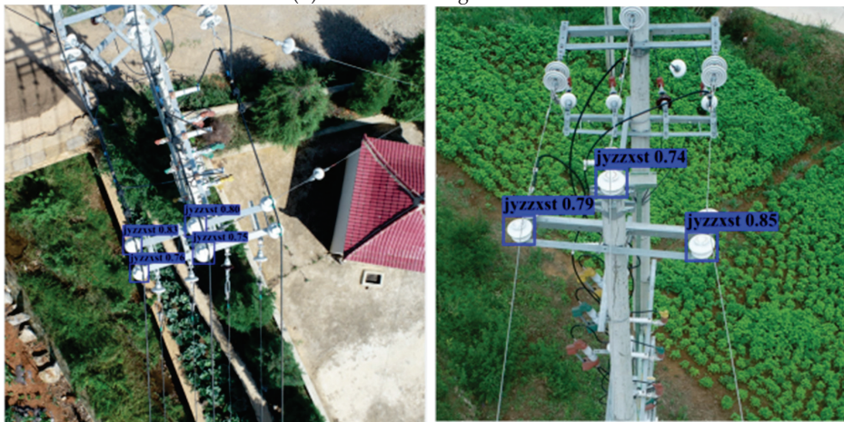
(c) Insulator tie wire loosening test results
