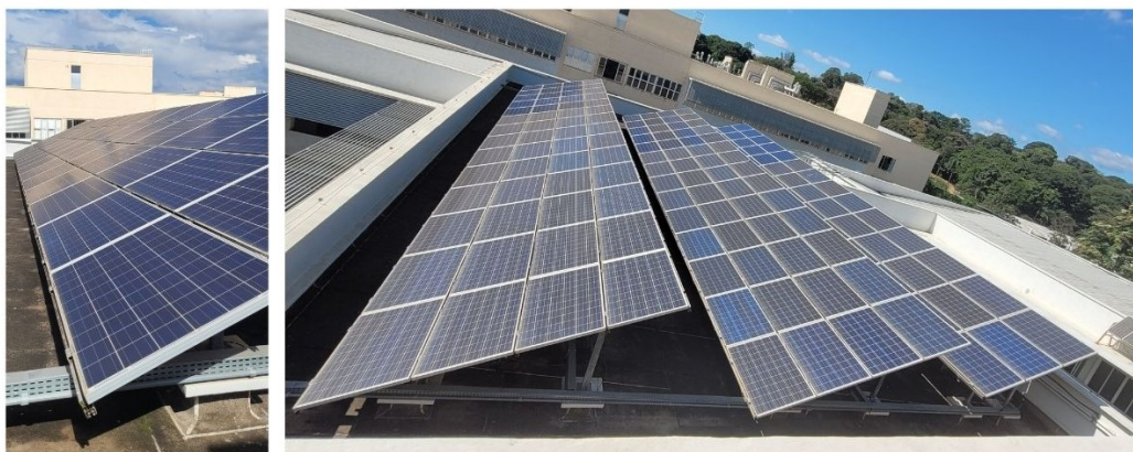
Figure 4. TESLA power engineering PV experimental plant.
