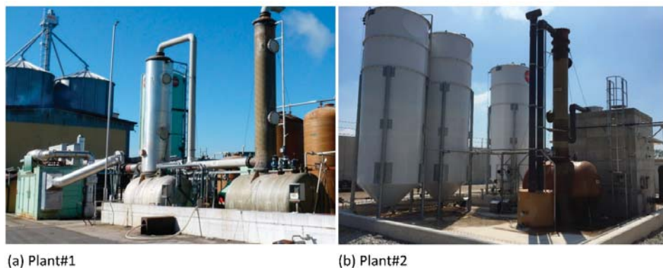
Figure 2. Ammonia recovery sections of plant #1 (a) and plant #2 (b).
