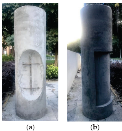
Figure 23. Concrete column with surface defects. (a) Hole. (b) Spalling.
