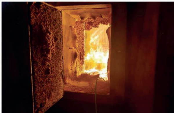
Figure 4. The middle part of grate—view from the middle inspection door of the boiler.
