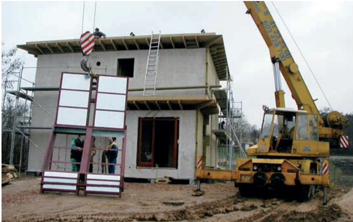
Figure 8. Installation of an experimental solar chimney on the roof of a demonstration house with a hybrid ventilation system.
