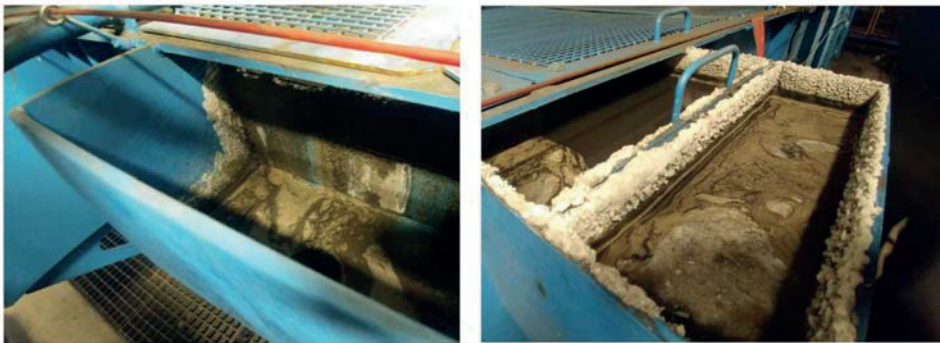
Figure 6. Tribocorrosion traces on the walls of deslagger water trap occurred during operation with high temperature water in the tub.
