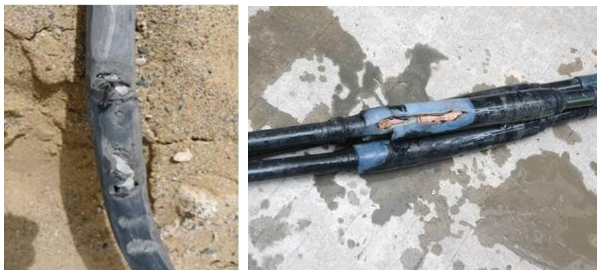
Figure 1. Insulation damage caused by overheating and moisture.
