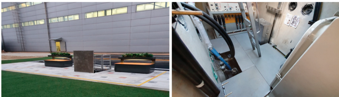
Figure 2. S-substation in Korea.
