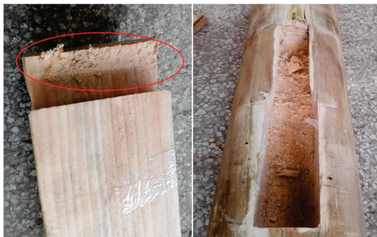
Figure 9. Wear of dovetail tenons and mortises.
