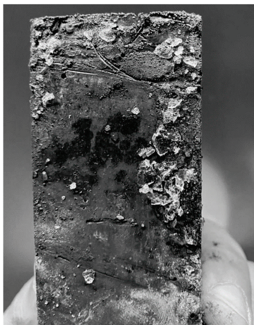
Figure 7. Efflorescence caused by \text{Na}_2\text{CO}_3 on the surface of a mortar specimen.
