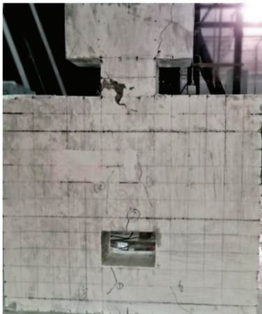
Figure 15. Failure condition of specimen ZZJ.
