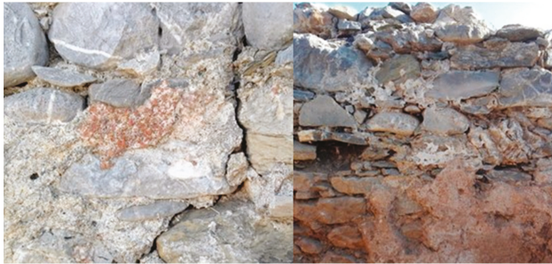
Figure 13. Details of hydraulic mortar covering both the outside and the inside surfaces at both bath-houses. (Photos: A. Tantsis).
