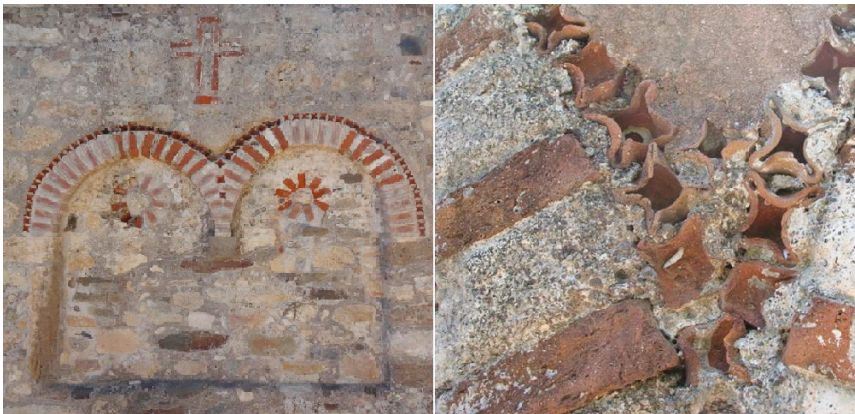
Figure 19. Detail of brickwork and rosettes on the facades of the Kato Episkopi Siteias church (bath-house). (Photo: A. Tantsis).
