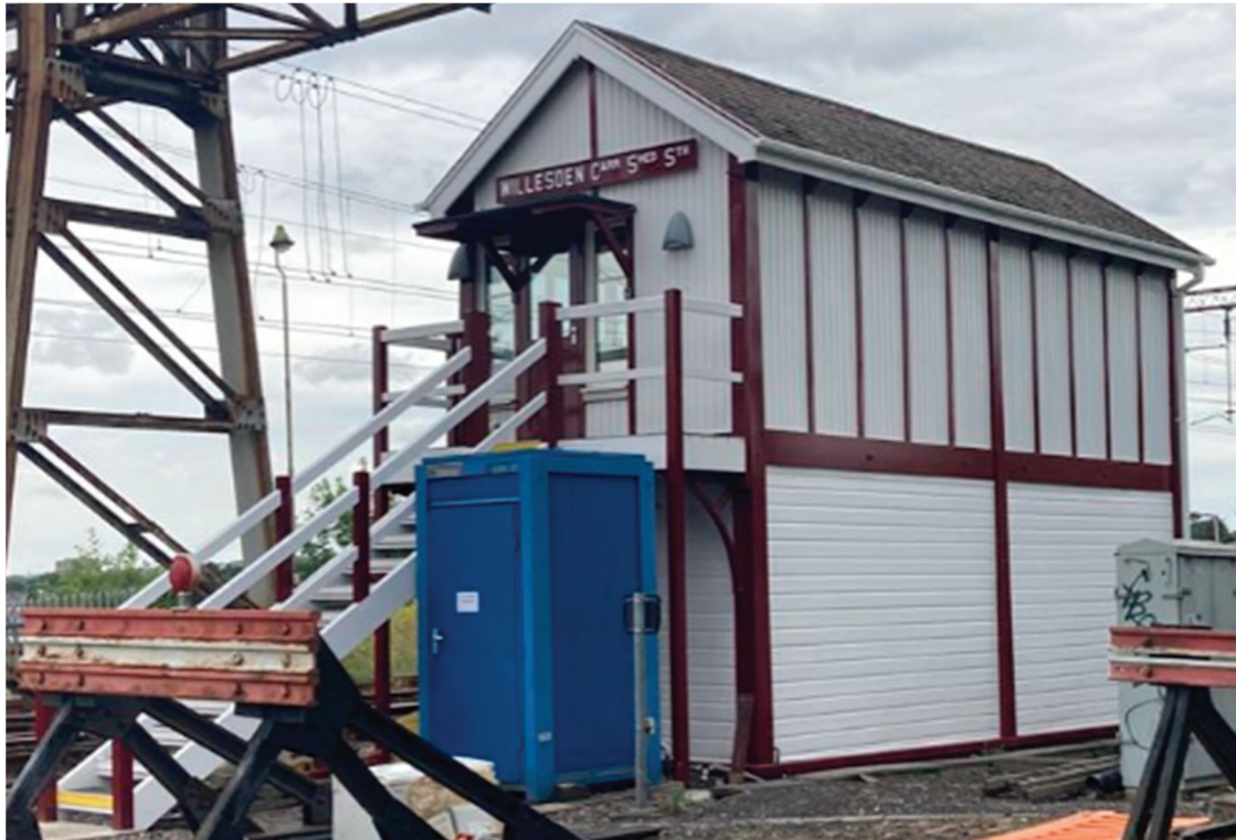
Figure 9. Drawings of approved repairs for the signal box and on-site application of the new cladding system.
