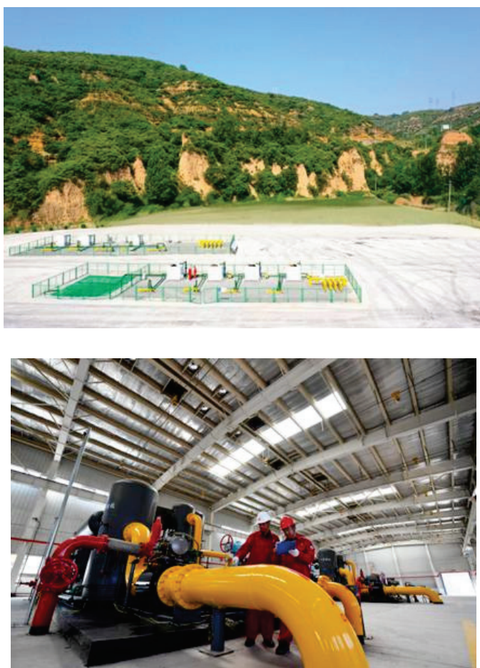
Figure 8. Field operation view and inspection/maintenance of CBM facilities in the Qinshui Basin, China.
