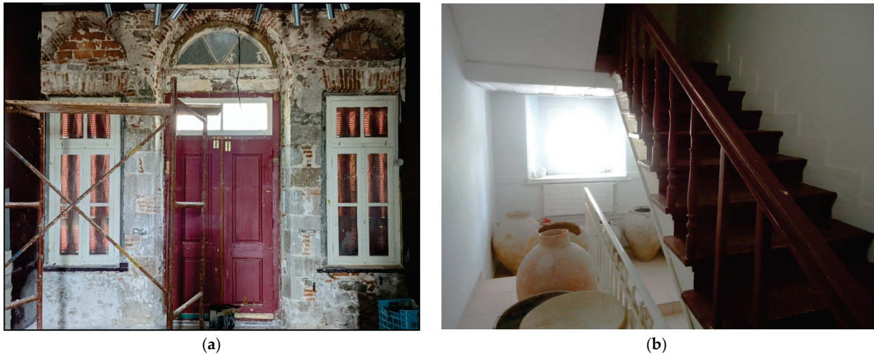
Figure 6. Structural features of the AML building: (a) Interior view of the external wall at the first level; (b) The two internal staircases of the building—a reinforced concrete staircase at the ground floor and a wooden staircase at the first floor. (Source: Digital Archive of the Ephorate of Antiquities of Lesvos, Hellenic Ministry of Culture and Sports; used with permission, Prot. No. 252765/16-06-2025).
