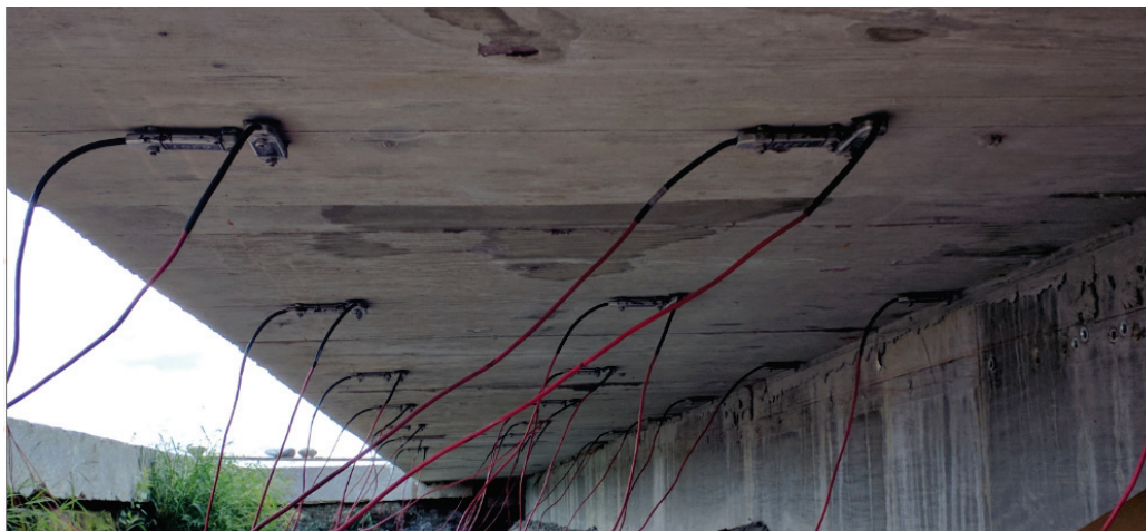
Figure 2. Sensors installed on the underside of the bridge deck for structural health monitoring.
