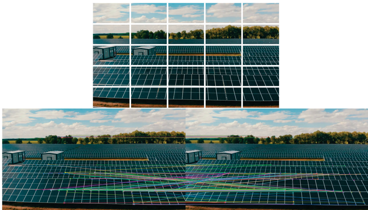
Figure 1. Photovoltaic power plant scene images.
