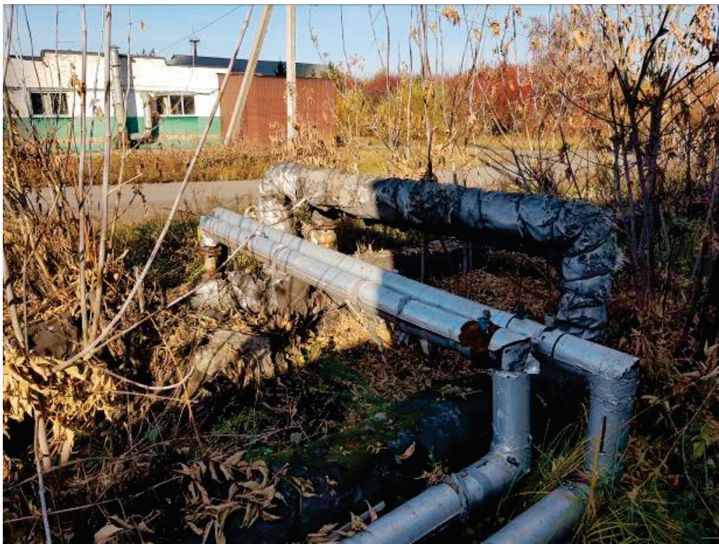
Figure 4. An example of high distribution heat losses due to poor insulation.
