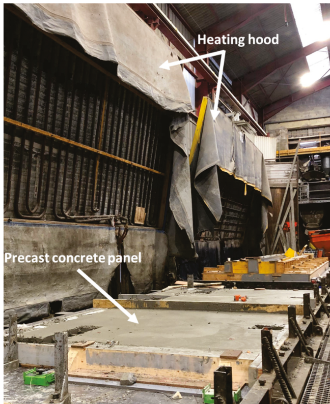
Figure 2. Heated hood system in precast factory.
