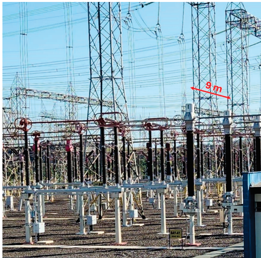
Figure 5. The 9 m distance between phases at the 500 kV Tucuruí Substation.
