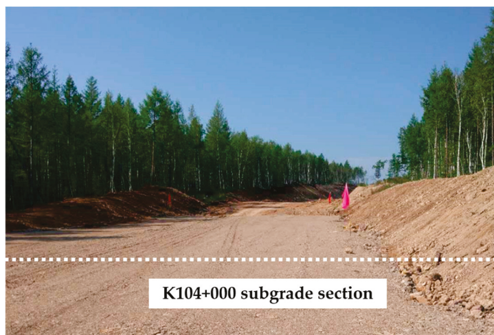
Figure 2. Actual scene of the K104+000 subgrade section.
