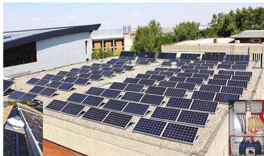
Figure 2. Roof-mounted 23.7 kW at 1000 W/m 2 and 25 °C multi-string PV system containing 95 CSUN250-72M modules (five parallel connected strings of 19 series modules; with adjustable tilt angles of 15°, 30°, 45° and 60°); coordinates 39.890917, 32.782278; five modules in the photograph are idle; terminal box of the system inside the laboratory is shown at the right bottom corner of photograph while the pyranometer is at left bottom corner.
