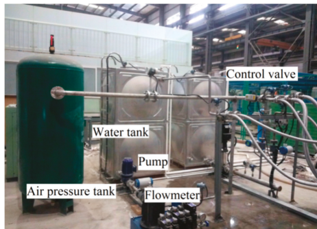
Figure 2. Air-water spray system.
