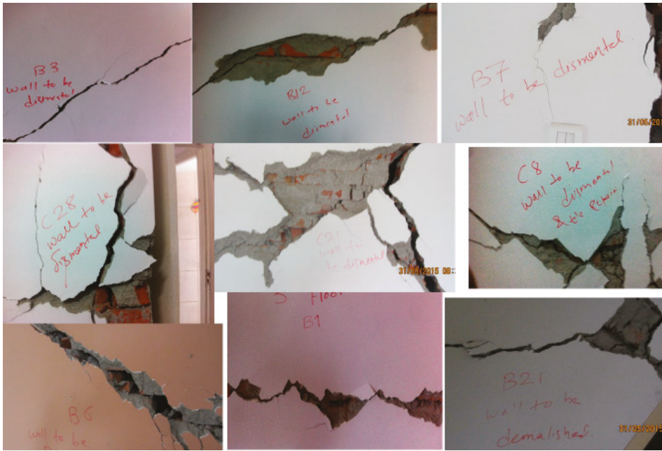
Figure 6. Infill wall damage due to Gorkha earthquake in the case study building.
