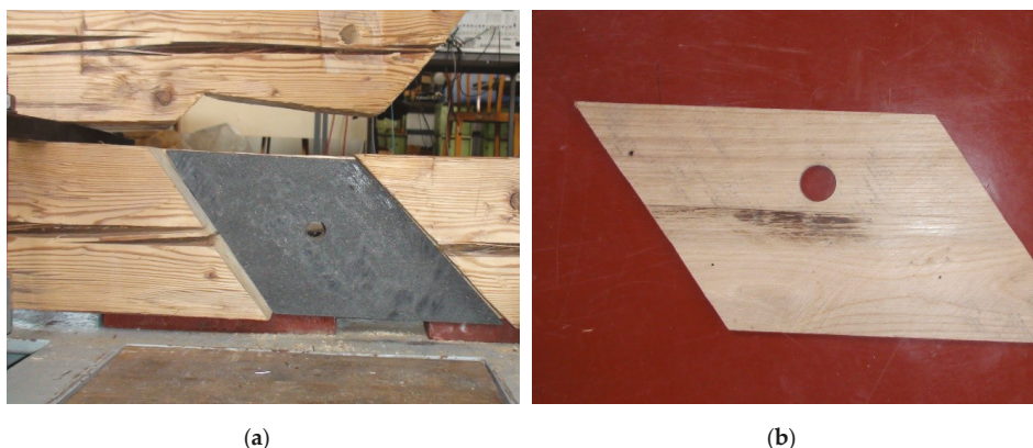
Figure 5. (a) Joint retrofitting with brake friction plate and replacement of the oak pin by a pre-stressed steel screw bolt; (b) an oak plate for joint retrofitting with friction plates.
