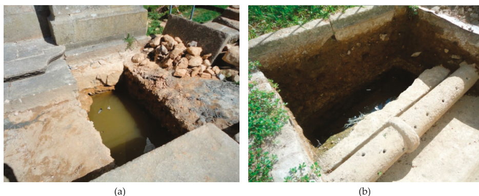
Figure 6. Water table visible in the inspection trenches days after the excavation (summer period). (a) Excavation 1: water level at -0.93 m below the nave floor; (b) Excavation 3: water table at -1.10 m measured from the floor of the nave.
