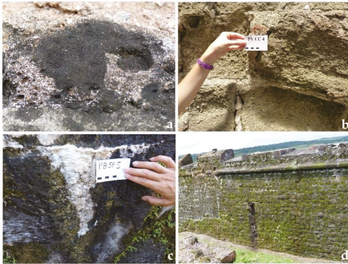
Figure 4. Pictures representing several deterioration processes observed at the sites. (a,b) at Panamá Viejo, (a) biological growth; (b) surface recession/material loss; (c) encrustation at Fort San Fernando (Portobelo); (d) biological growth at Fort San Lorenzo.
