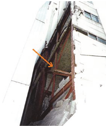
Figure 1. Diagonal brace collapsed in the 1995 Hyogoken Nanbu earthquake [23].
