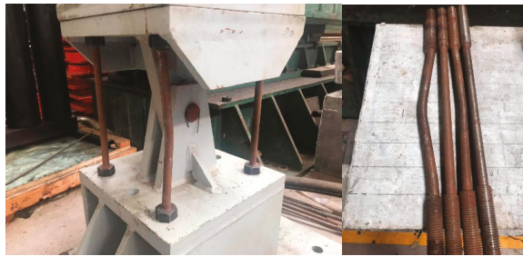
Figure 14. Bolt failure pattern.
