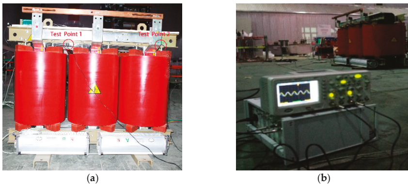
Figure 2. (a) Position of vibration-acceleration sensor; (b) field experiment.
