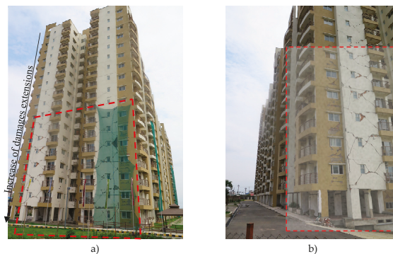
Figure 5. Survey damage assessment of the building: (a) north façade; (b) south-east façade.
