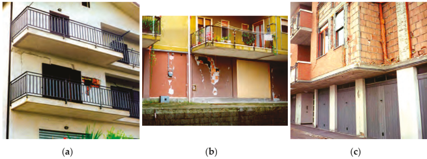
Figure 2. Examples of Medium-Severe and Very Heavy damage to infills: horizontal and vertical cracks between infill and beams/columns—widespread damage D2–D3 and locally D4–D5 (a); damage D4–D5 to infills (b); damage D4–D5 with out-of-plane collapse of one infill leaf (c)—adapted from [4].
