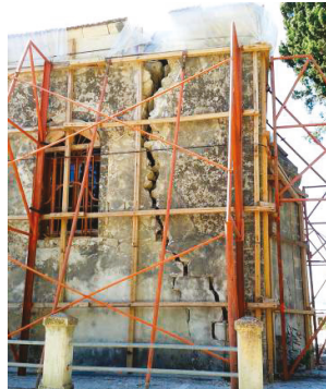
Figure 18. Damage at the N-W corner.
