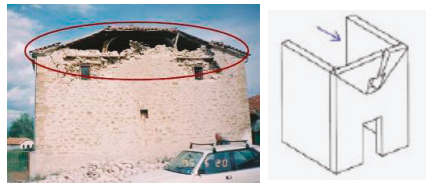
Figure 8. Typical out-of-plane damage of longitudinal wall. Kozani-Greece Earthquake 1995.
