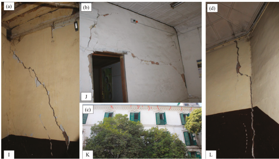
Figure 5. Local damages in the monument (a) diagonal crack on the third-floor wall, (b) horizontal and vertical cracks beside the opening, (c) exterior wall damage at the top floor, (d) corner damage (uppercase indications at the bottom of the structures are the location indications as shown in Figure 2).
