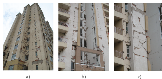
Figure 1. Fourteen-storey reinforced concrete structure damaged after the Gorkha earthquake: (a) distribution of the damages from the first to the seventh storey; (b) detachment of the walls from the envelope frame; (c) diagonal cracking with slight out-of-plane detachment of the wall.
