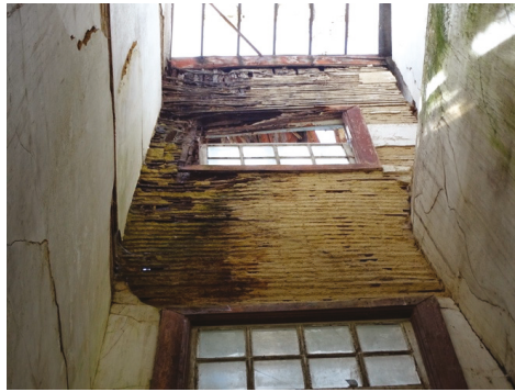
Figure 7. Severely decayed structural elements.
