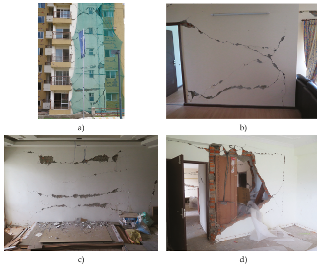
Figure 6. Survey damage assessment of the interior of the building: (a) diagonal cracking in façade wall; (b) diagonal cracking in interior partition wall; (c) sliding cracking in interior partition wall of storey 1; and (d) out-of-plane collapse of interior partition wall.
