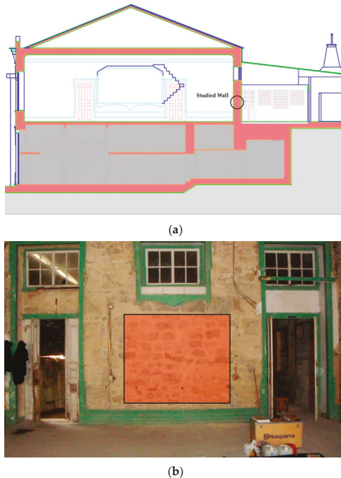
Figure 5. Identification of the studied wall. (a) location in the building; (b) testing area.
