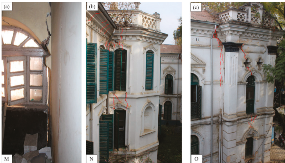
Figure 6. Local damages in the monument (a) corner damage, (b) corner damage and crack propagation in the projection part, (c) cracks developed above the arch. In figure, uppercase indications at the bottom of the structures are the location indications as shown in Figure 2.
