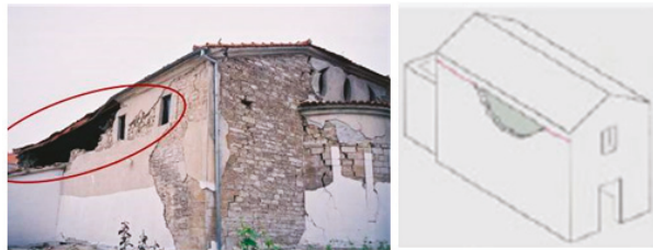
Figure 7. Typical out-of-plane damage of longitudinal wall. Kozani-Greece Earthquake 1995.
