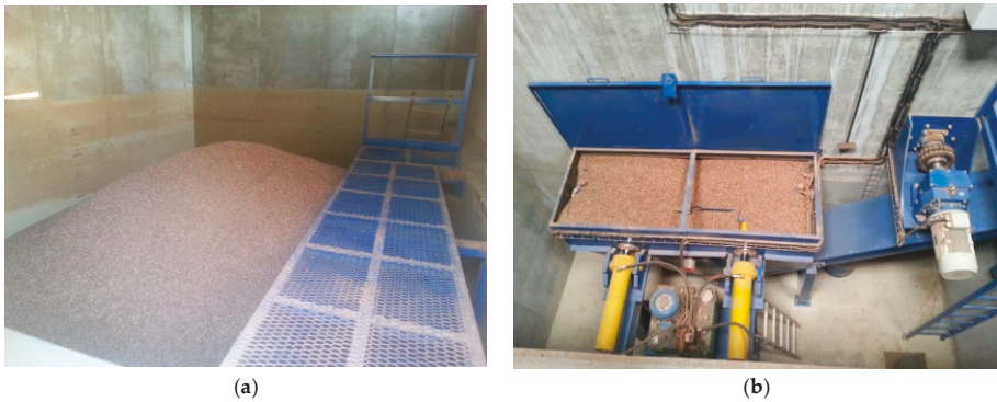
Figure 8. Biomass warehouse (a) with a burner automatic feeding system (b).
