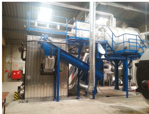
Figure 7. Example of a biomass burner in a steam boiler of a textile production plant.
