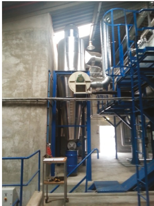
Figure 9. Biomass steam boiler filtering system.
