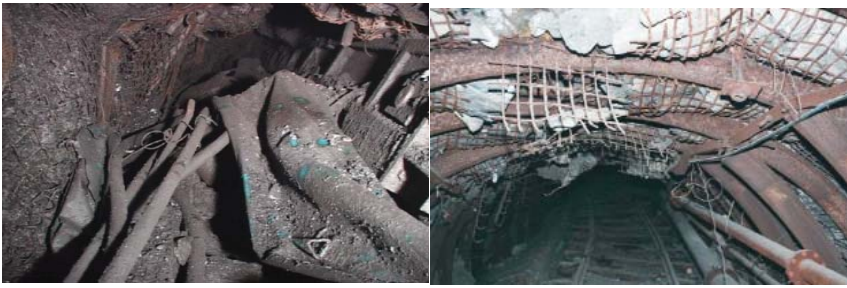
Figure 1. Field photos after severe roadway damage.
