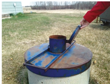
Figure 3. Cistern cap, intact but unlocked. Photo credit: R. Patrick.
