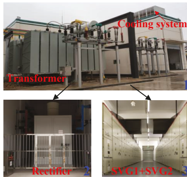
Figure 13. Low-harmonic DC ice-melting device in 35 kV Chuanshan substation.
