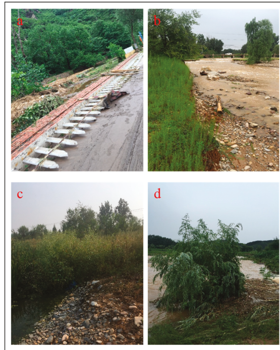
Figure 1. The protection measures damaged by the flood. (a) Destroyed retaining wall; (b) collapsed riverbank; (c) the living brush mattress measure before the flood; (d) the living brush mattress measure during the flood.
