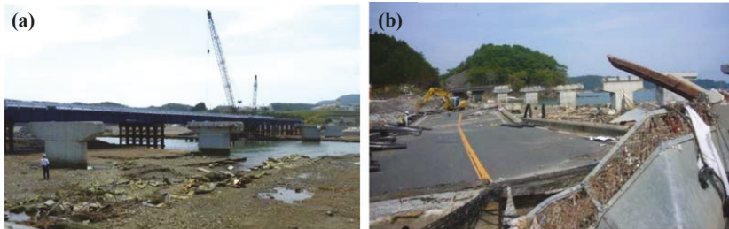
Figure 1. Damaged bridges after the 2011 Great East Japan Earthquake: (a) Koizumi bridge on the left (photo: E. Monzon) and (b) Utsu Bridge on the right (photo: I. G. Buckle).
