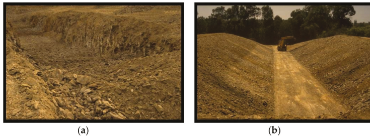
Figure 3. (a) Excavation of the mica schist ground support; (b) shape of the test site between embankments.
