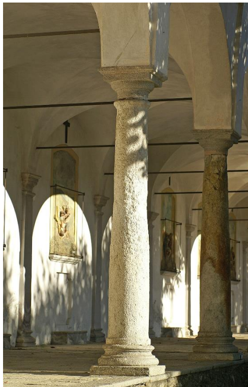
Figure 2. The stone columns of the Via Crucis portico in the Sacro Monte at Ghiffa.
