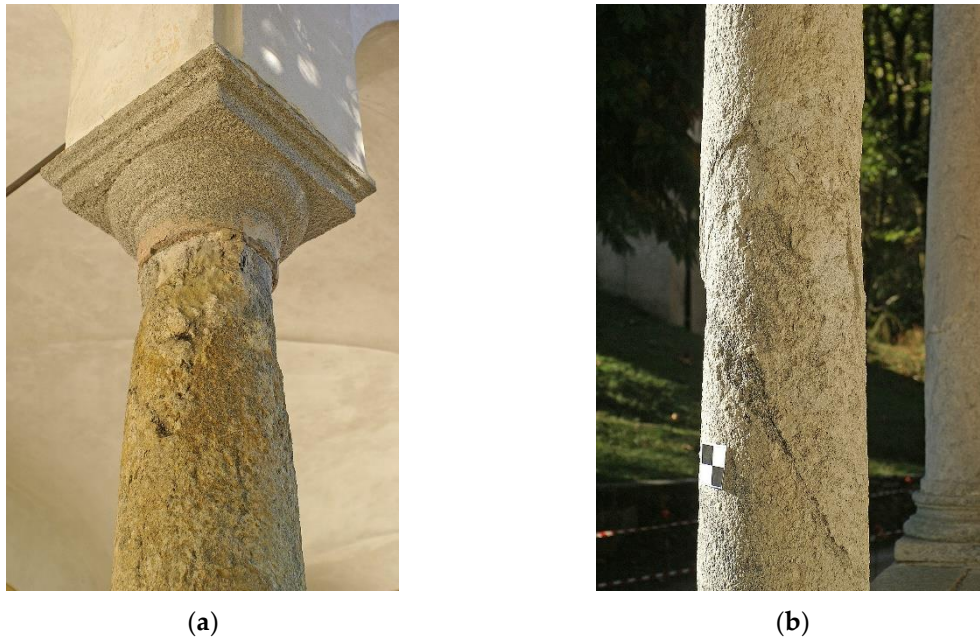
Figure 7. Different types of surface material degradation on the columns of the Via Crucis portico: (a) erosion; (b) exfoliation.
