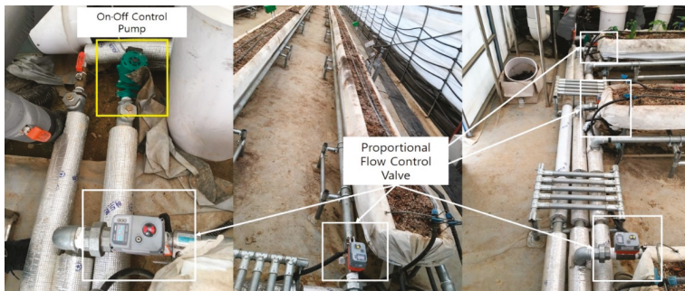
Figure 16. Images of the pump and valves installation for heating control in greenhouse B (Case 2).
