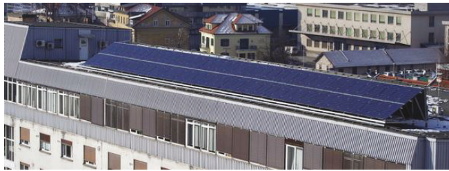
Figure 6. LPVO PV system on the roof of Faculty of Electrical Engineering in Ljubljana.
